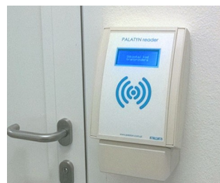
RFID access control readers
