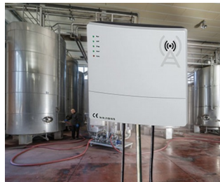
Gateway for the automation of production plants
